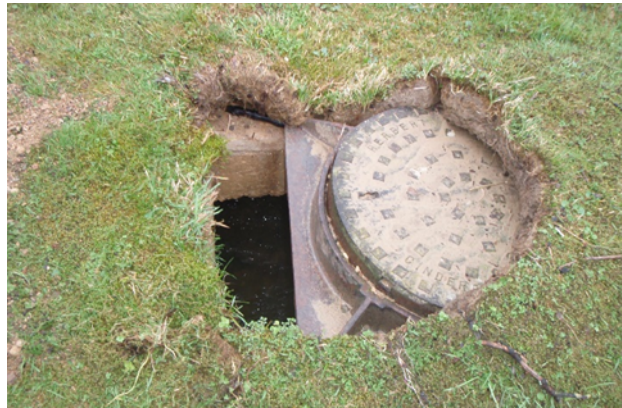
Photograph 6-1 Manhole located along Dog Lane which lifts under high flow conditions
